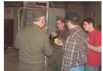
Shawn Welch, Jonathan Prostak, Mike Murray and Stephen Turner working on the BD-74 Fire Control Switchboard.
