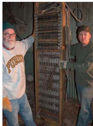
Leo Polaski and Andy Grant working on recovering one of the BD-74 Fire Control Switchboards from Fort H.G. Wright.
