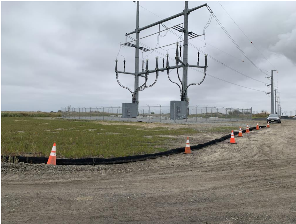
Photo looking northeast towards the recently constructed Silver Run H-frame/overhead transmission
