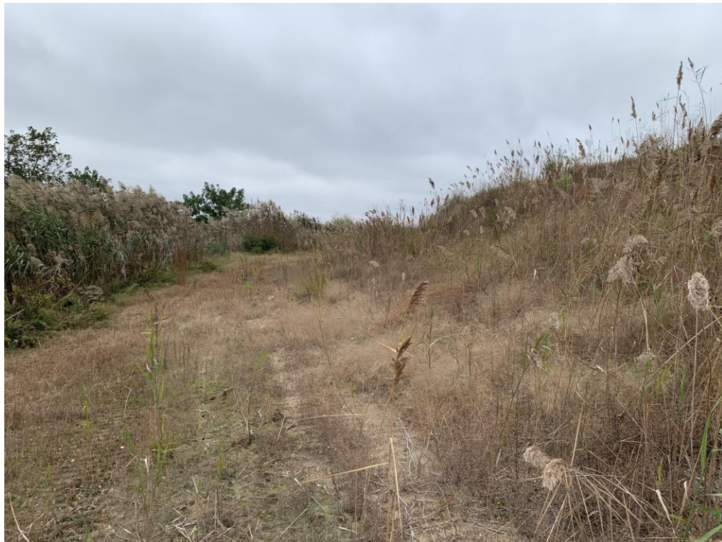
Photo looking southwest along the bottom of the USACE CDF Cell No.3 berm.
