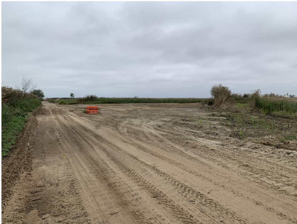
Photo looking northeast into the PSEG CDF.
