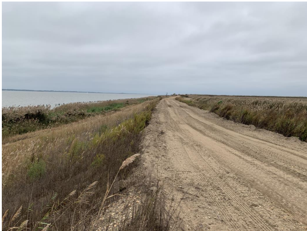
Photo looking north along the western berm of the USACE CDF Cell No.3. Photo taken standing on top of berm. Note Delaware River and shoreline coastal wetlands on the left.
