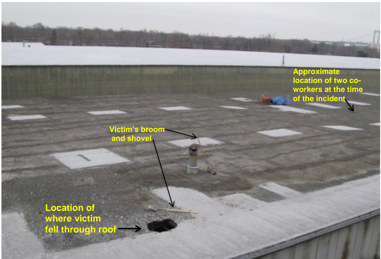
FIGURE 2. Scene at time of incident with location of where victim fell through the roof.
