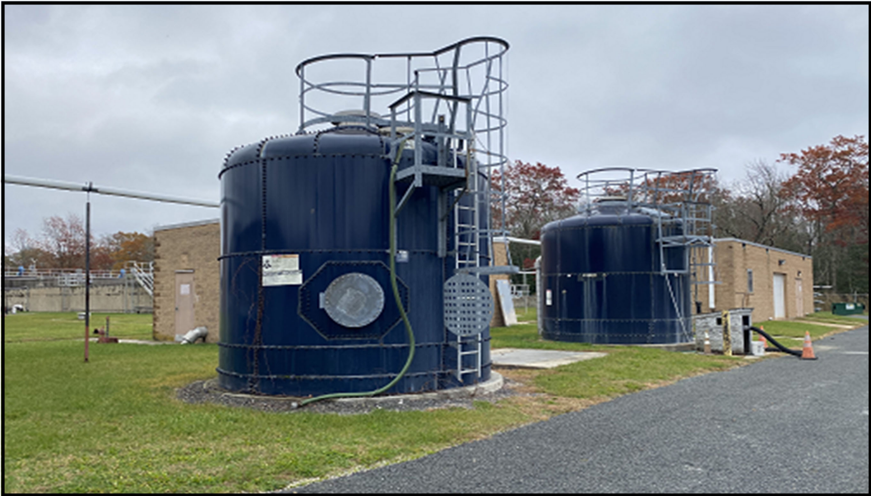
Photos - Sludge Storage Tanks Bayside State Prison - Waste Water Treatment Plant EXHIBIT 'C'
