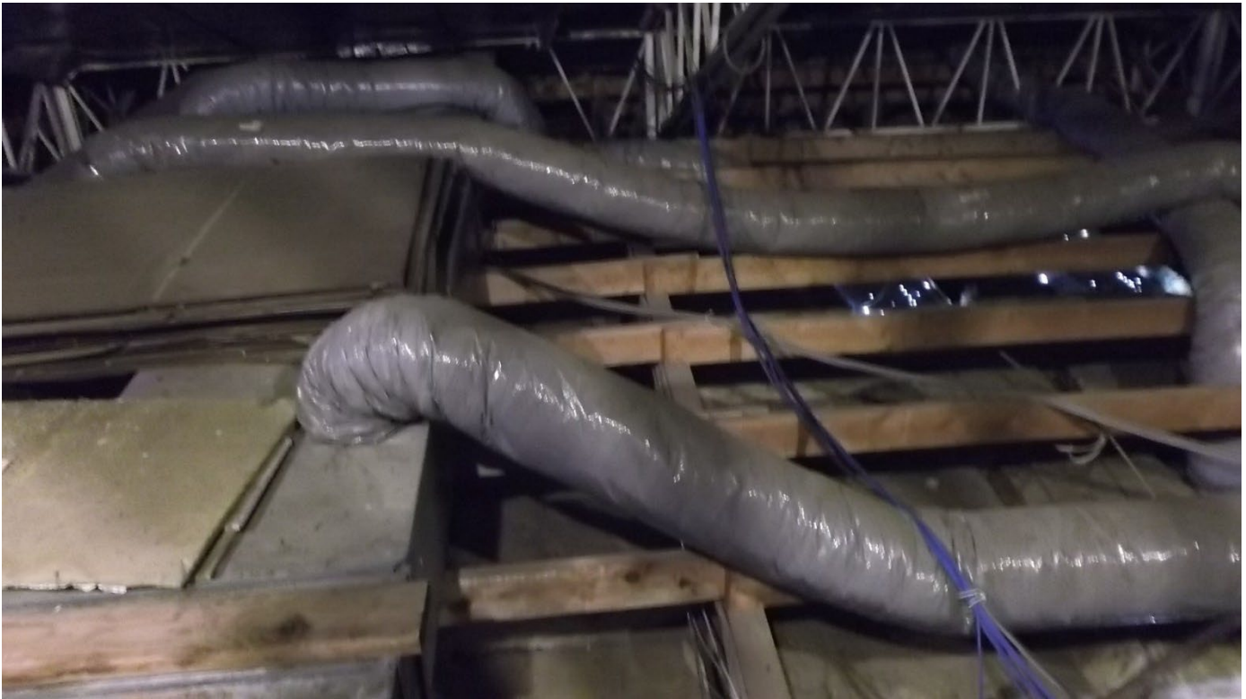
Fixed and flexible ductwork in central attic.
