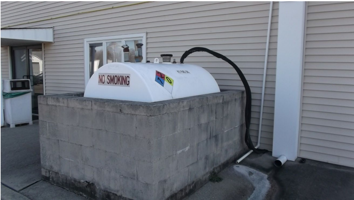
#2 Fuel Oil Tank.
