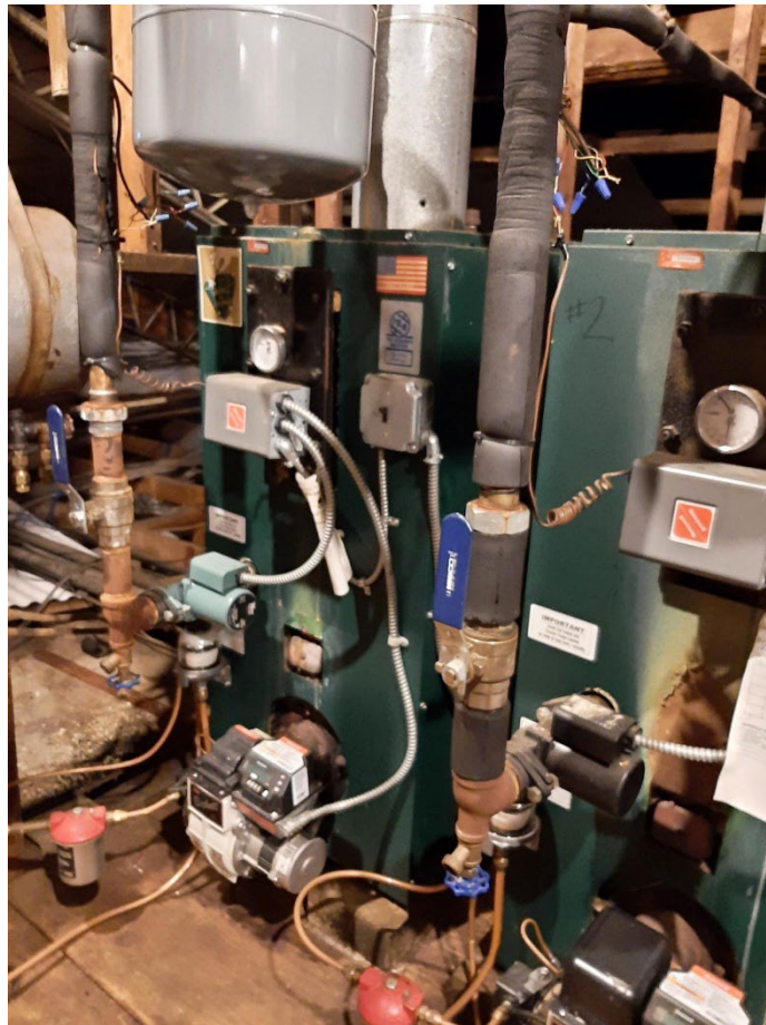
Two boilers side by side in central attic.
