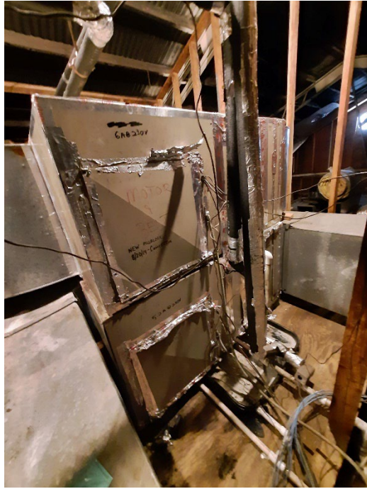
Air handler in central attic.
