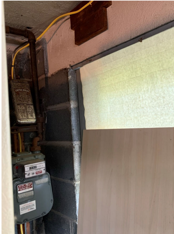
Photo 5. CMU Wall Along Front Wall of Garage, Timber Frame Wall Above Window
