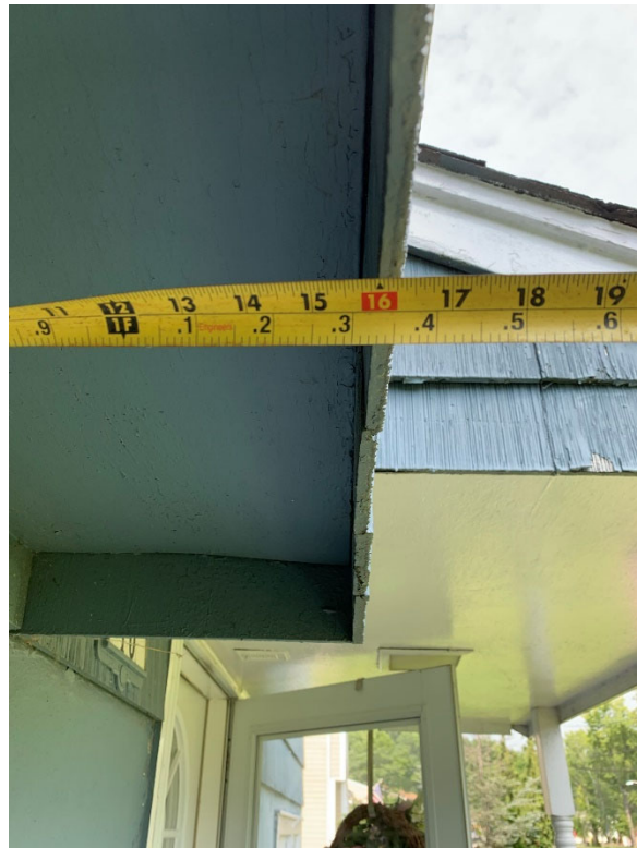
Photo 13. Second-Floor Overhang Over Garage Front Wall
