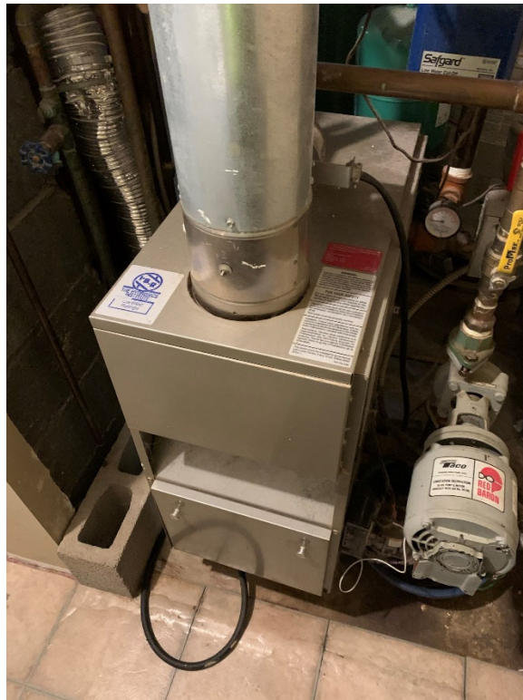
Photo 10. Boiler in Boiler Room (Looking North)
