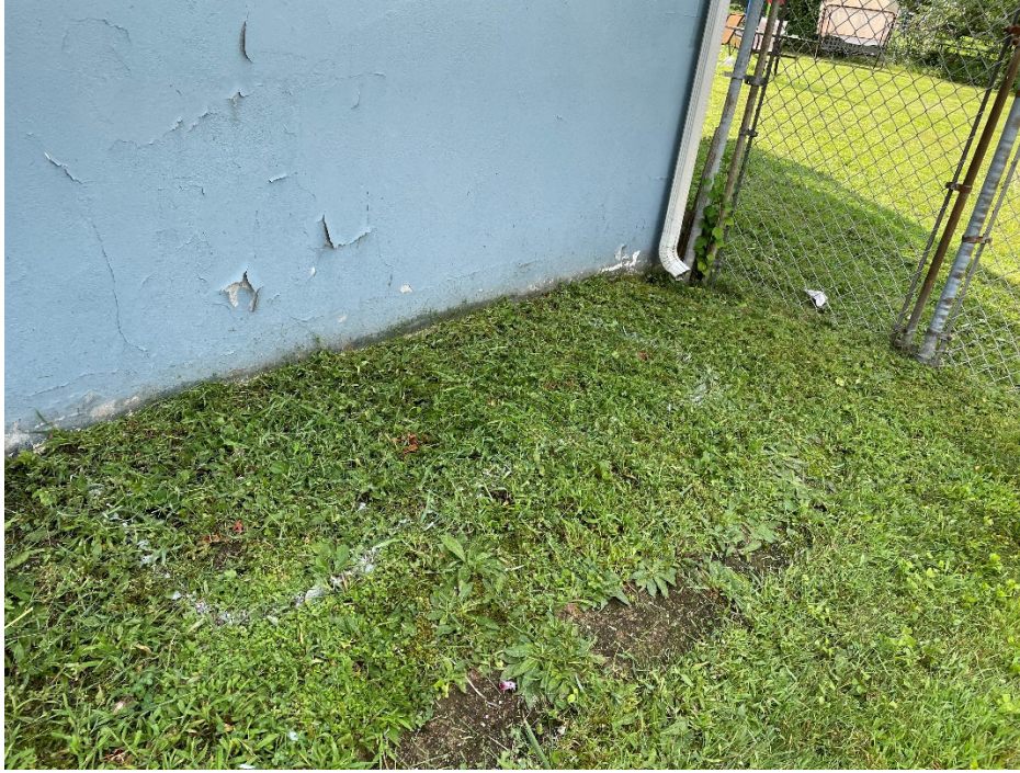
Photo 15. Test Pit TP-1 Location (Southwest Corner of Building – Ground Level Living Space)
