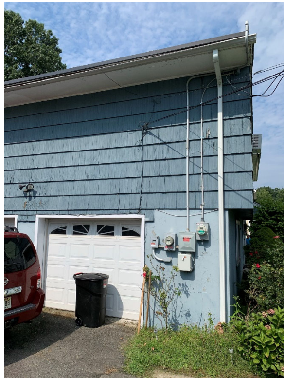
Photo 12. Solar Panel Equipment on East Exterior Wall of House
