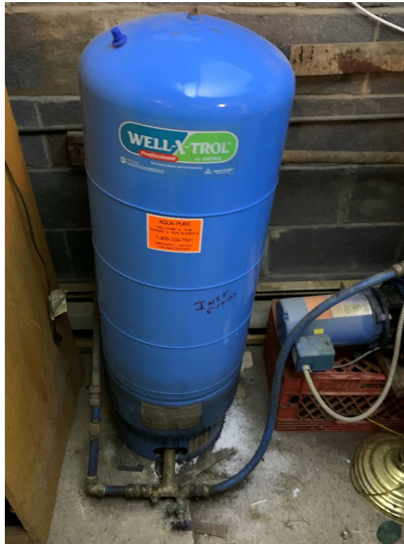
Photo 6. Water Well Pressure Tank & Pump, West Wall of Garage
