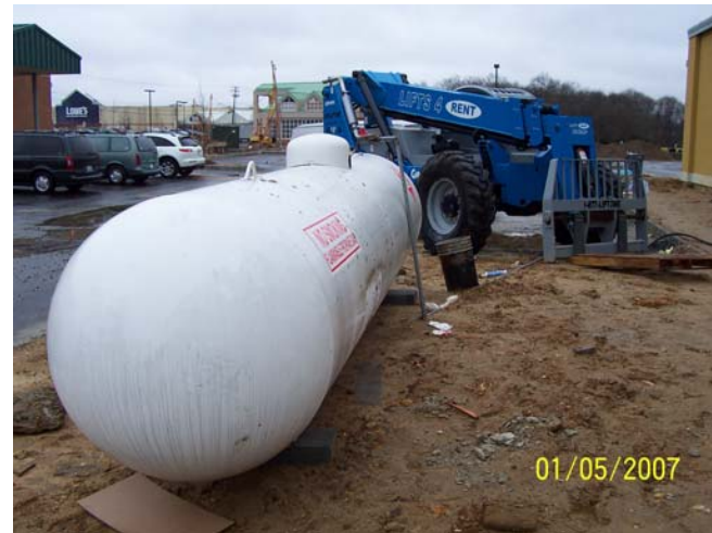
Tanks need to be placed on firm stable earth and be protected from construction vehicle traffic
