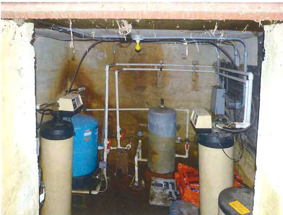
NJ_BURLINGTON_RIDGWAY, HOUSE, WILLIAM_0053 View facing south in the pump house.
