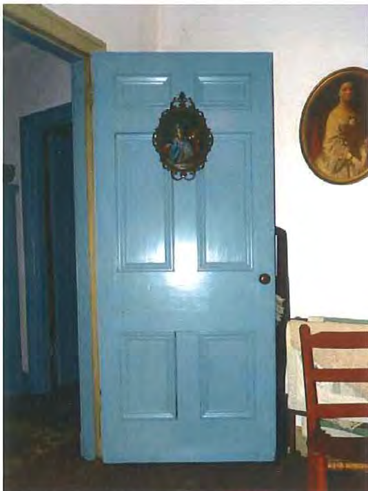
NJ_BURLINGTON_RIDGWAY, HOUSE, WILLIAM_0037 Detail facing southeast in room 303 showing a typical third floor door.
