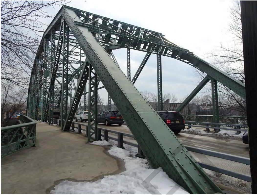
Straight Street Bridge over the Passaic River, City of Paterson, Passaic County Photo #3
