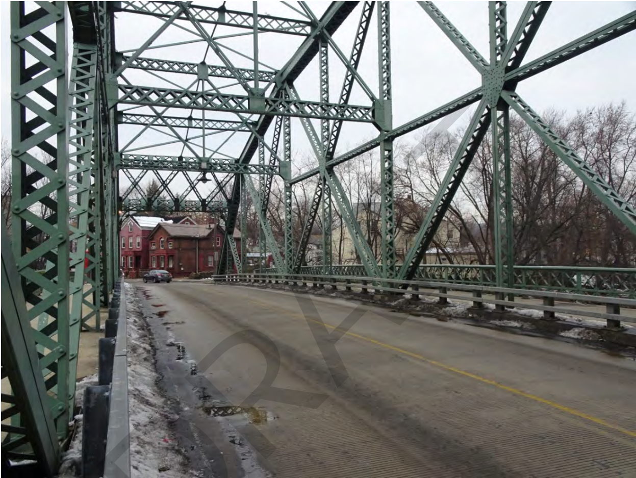
Photograph 9. View of truss work and deck, looking northwest toward North Straight Street.
