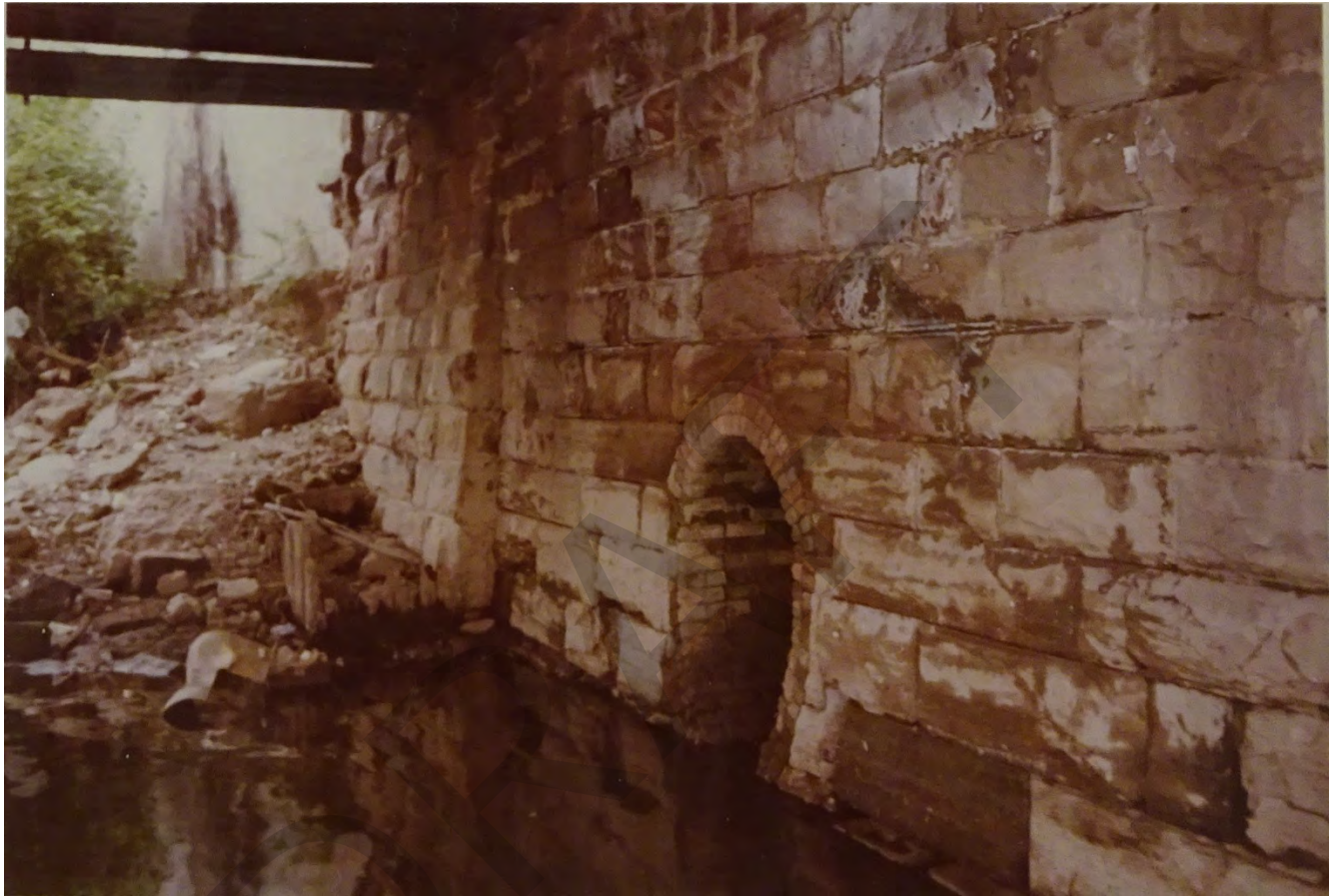
Figure 5. A 1979 photo showing the stone south abutment remaining from the second Straight Street Bridge, before repairs were made.
