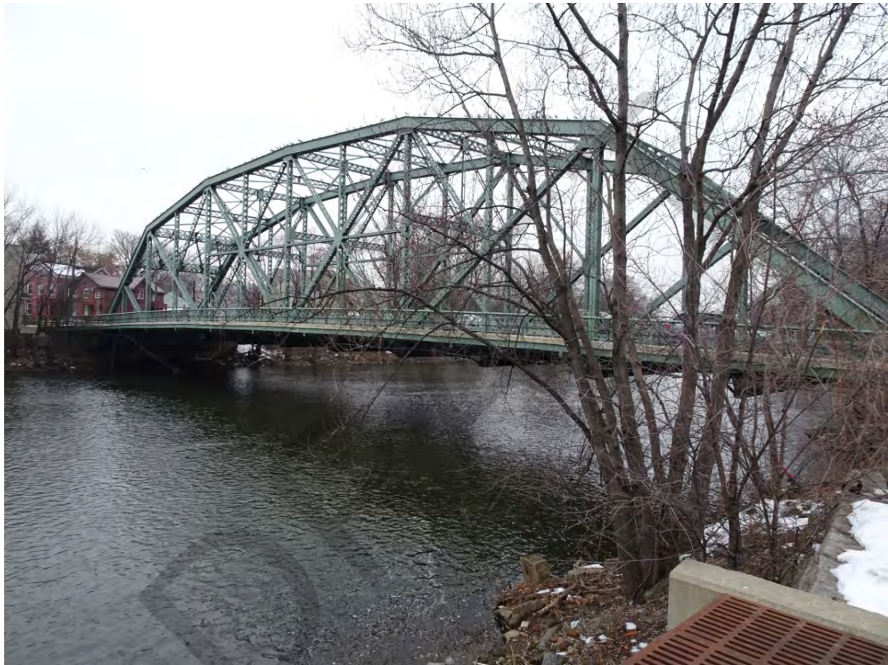
Photograph 1. View north from the river banks at River Street, looking toward the southwest elevation of the bridge.
