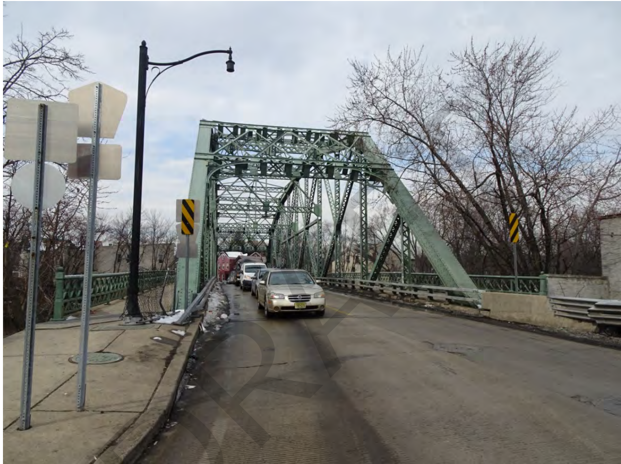
Photograph 2. View of the bridge deck from the River Street and Straight Street approach, looking northwest.
