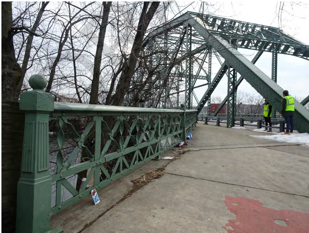
Straight Street Bridge over the Passaic River, City of Paterson, Passaic County Photo #6
