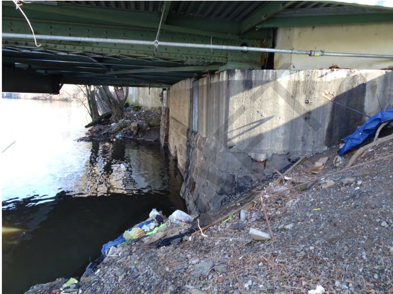
Photograph 14. View of south abutment with masonry of earlier span below and reinforced concrete above, looking northeast.
