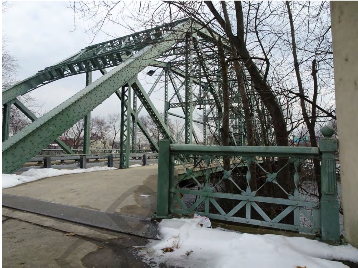
Photograph 12. View of the bridge and pedestrian railing from the North Straight Street approach, looking southeast.
