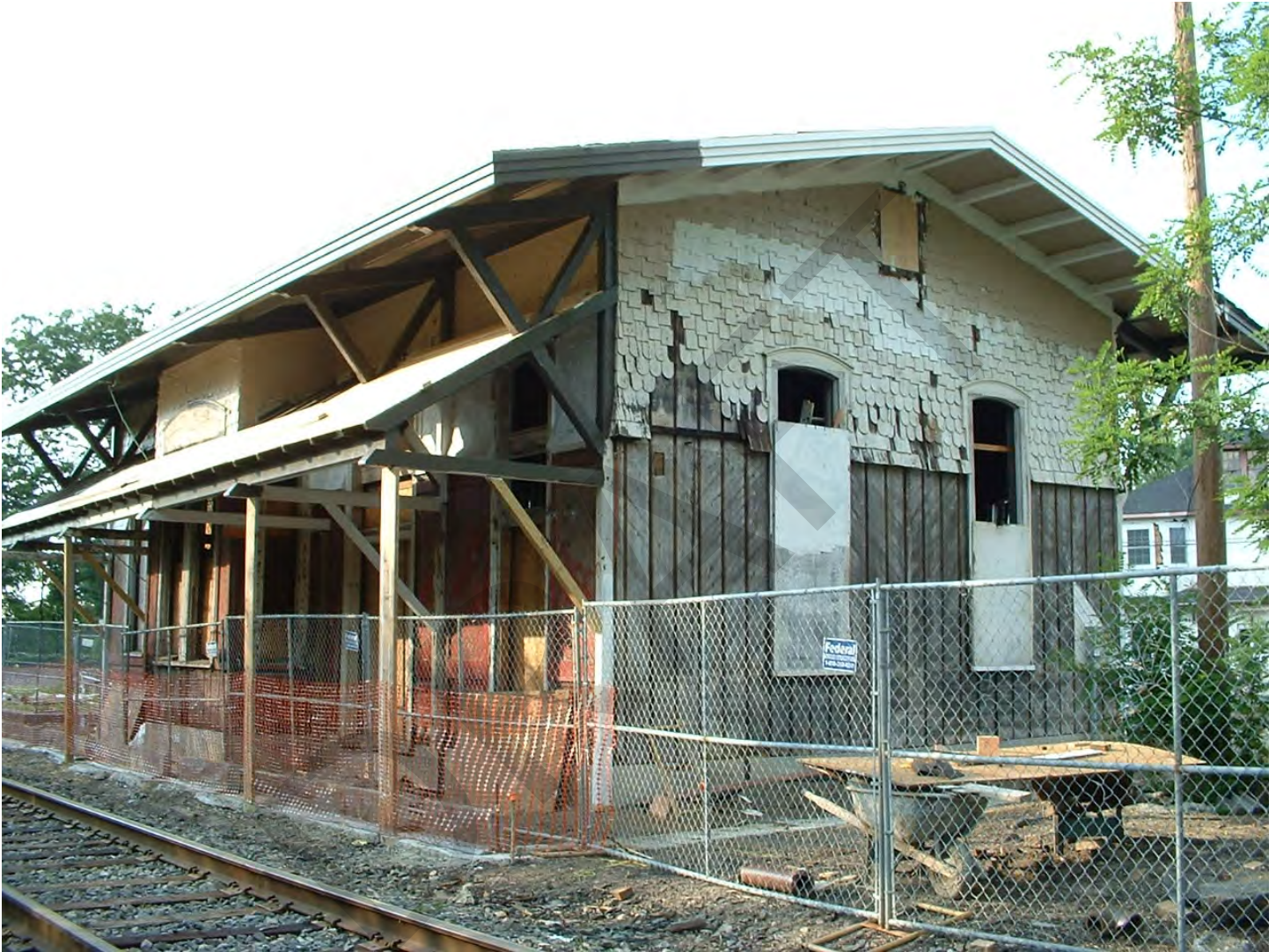
View of the west and south elevations during the 2014 restoration, showing the vertical boards of the original board-and-batten siding.
