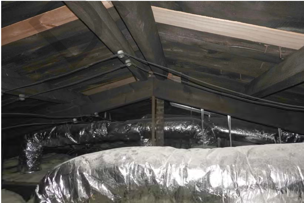
Photograph 0027: Attic space looking north from the south end, showing solid board roof sheathing, through-purlins, and the top diagonal chords of the king rod truss.
