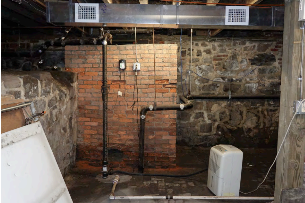
Photograph 0024: Interior view from the basement entry, camera facing west, showing the 1892 brick coal bin, and the crawlspace at left (south).
