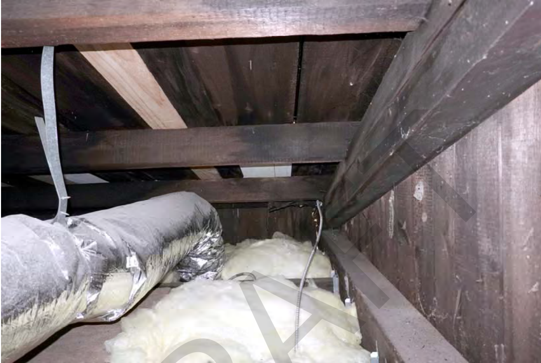
Photograph 0026: Attic view, looking east along the south gable end wall, showing the interior face of the original board siding and the bottom and diagonal chords of Truss #1.
