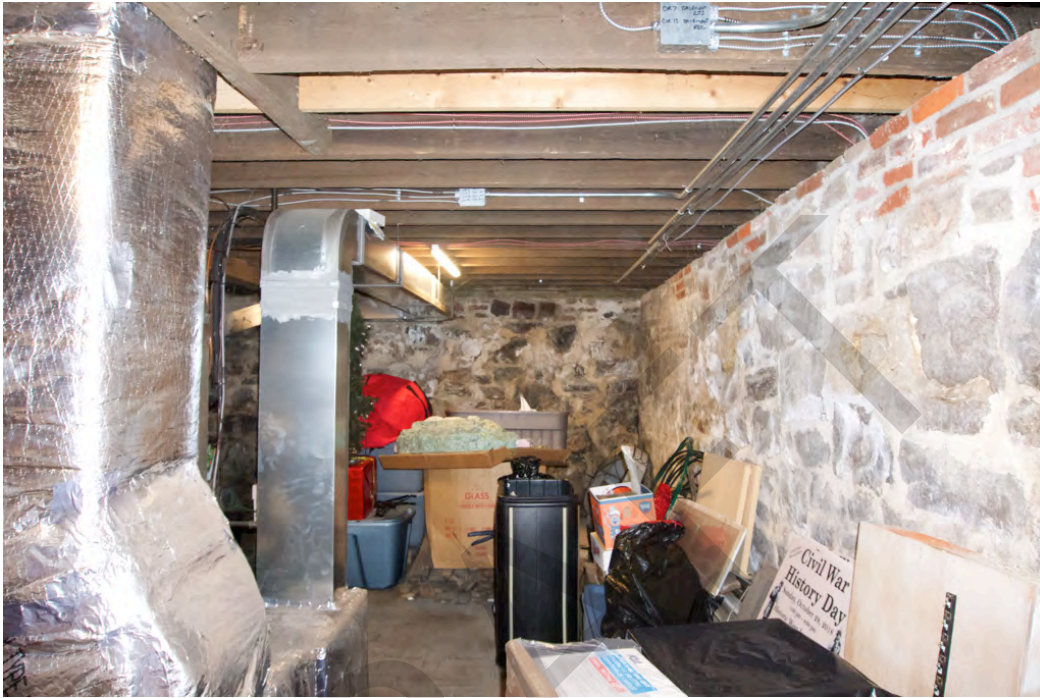
Photograph 0022: Interior view of the basement, camera facing north, showing the 1892 stone and brick walls.
