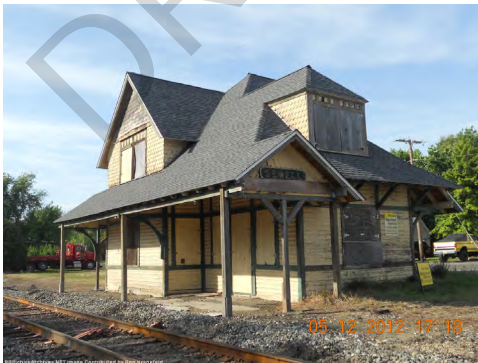
Supplemental Photograph 15: Sewell Depot (c.1885), WJRR. Note the stickwork and use of drop siding and half-cove shingles. Note also the different building form.
