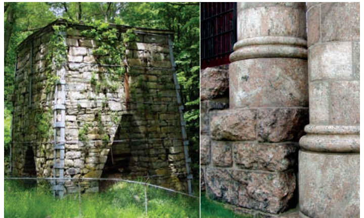
Figure 5. Examples of granite's use as a building stone: Wawayanda furnace ( left ), Wawayanda State Park, Vernon Twp., Sussex County, and St. Paul's Episcopal Church ( right ), Paterson City, Passaic County. Photos by R.A. Volkert
