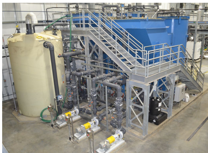
View of the metals precipitation phase of the groundwater treatment system.
