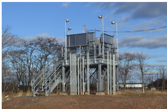
Critical system infrastructure was raised above historic flood levels to help build resiliency in storm events.
