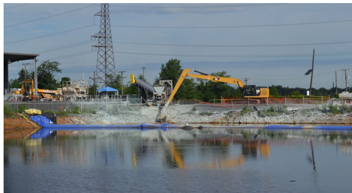
Remedy demonstrations were performed in 2020 and 2021 to gather information for the final design of the OU8 remedy.
