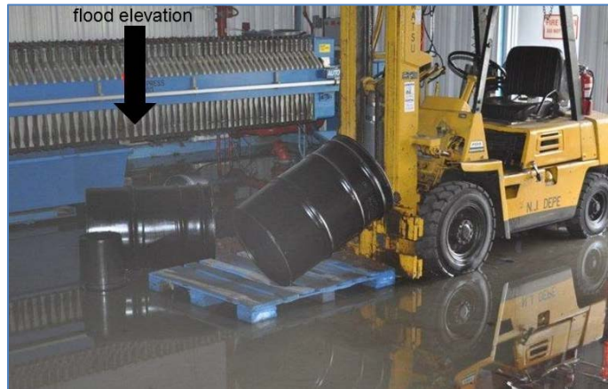
Figure 2-2 Flooding caused costly damage to mechanical and electrical equipment (courtesy Handex Consulting & Remediation, LLC).
