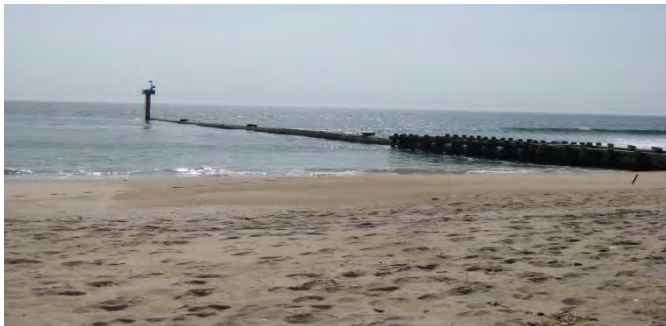
Stormwater outfall pipe (with extension), Atlantic Ocean side
