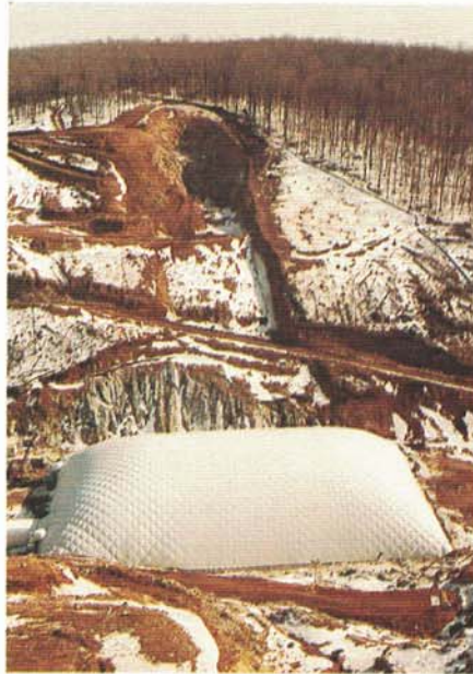
A heated dome was erected at the Merrill Creek construction site on Jan. 9, 1987 to enable work to continue on the $217 million project over the winter. The flexible, plastic-like structure covered about 53,000 square feet of the valley floor.
