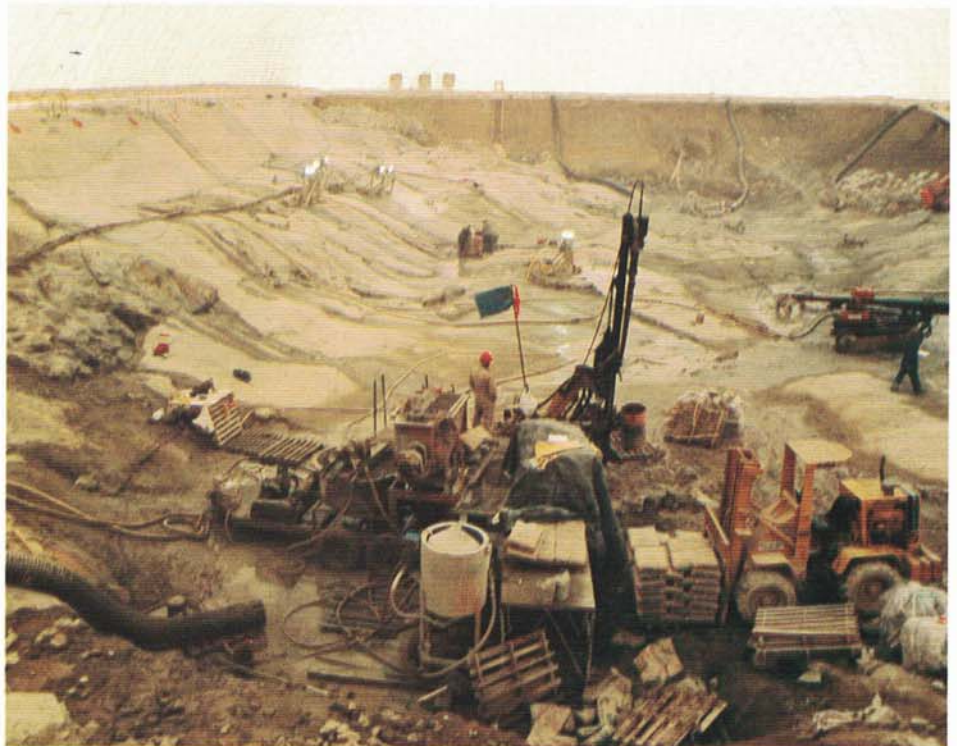
Air inside the dome was heated to 45 degrees making it possible to work with concrete and complete other tasks held up by inclement weather the previous year. The dome, which cost about $600,000 to erect, was removed in March of 1987.
