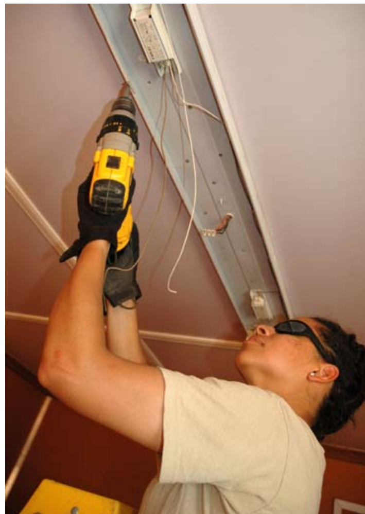
New Jersey Air Guard Staff Sgt. Anne McKenzie, an electrician, installs an overhead light fixture in a trailer her unit recently re-located at Baghdad International Airport. U.S. Air Force Photo by Master Sgt. Louis Conzo.
