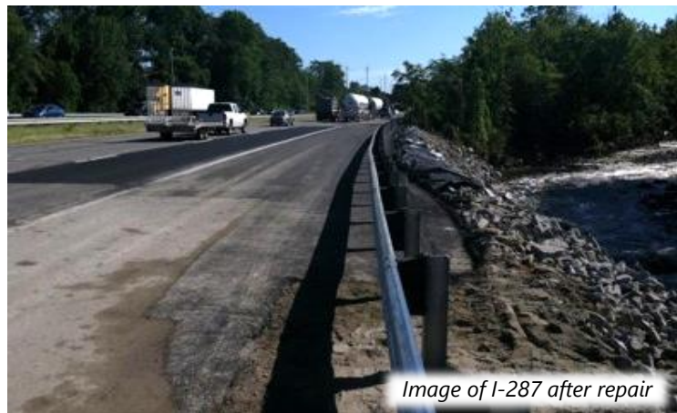
Image of I-287 after washout
