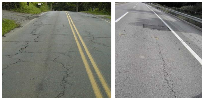
Exhibit 2-11: Block and Longitudinal Cracking
