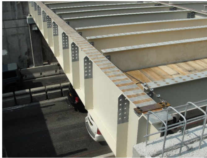
Exhibit 5-17: Galvanized Steel Girders with Painted Overcoat (Except at faying surfaces of the connections) – NJ Route 139
